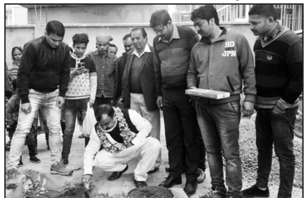
MLC, Vikram Randhawa laying foundation of drain at Shiv Shakti Mohalla, Narwal Bala on Saturday.
