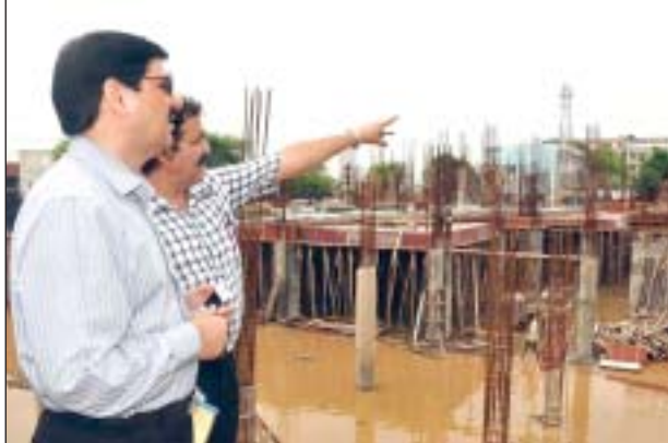
Minister for Law Mir Saifullah inspecting construction work of new Legislature Complex at Jammu on Thursday.
