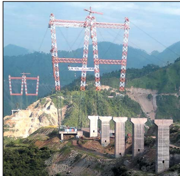
Cable cranes installed across river Chenab to facilitate erection of arch of upcoming world's highest Railway bridge.
