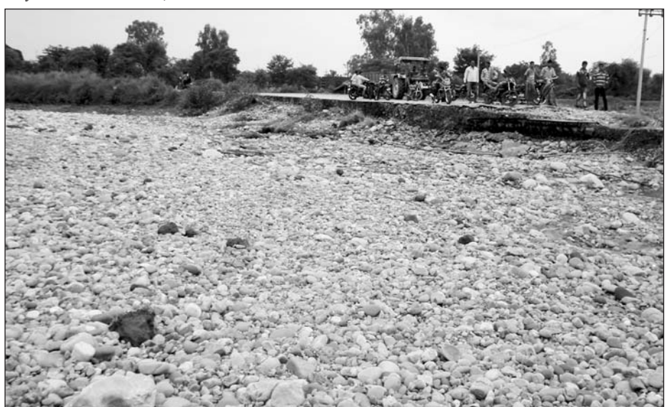
Nearly 70 mt portion of road washed away as 'bund' breaches at Sherpur on old Samba-Kathua road due to flood.
