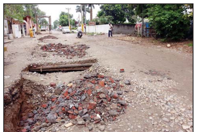
Dilapidated condition of road from Bakshi Nagar to AG office.
