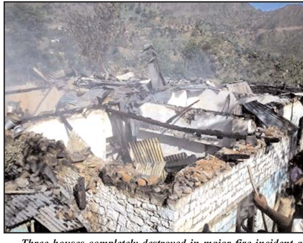
Three houses completely destroyed in major fire incident at Pathana Teer in Mendhar on Friday. -Excelsior/ Nazki
