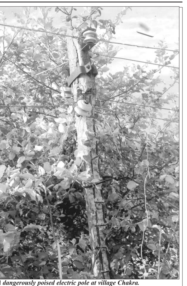
A dangerously poised electric pole at village Chakra.
