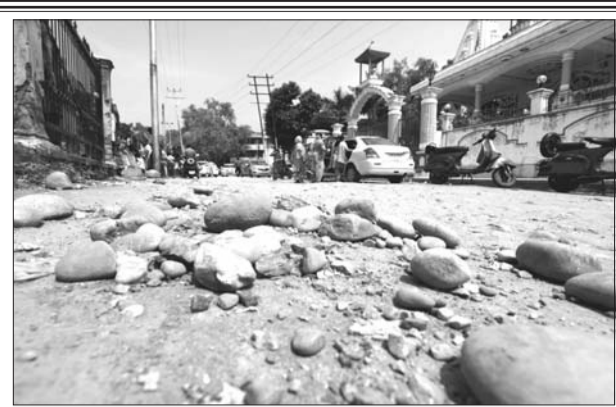
Canal road Opp. Shiv Dham temple in deplorable condition.
