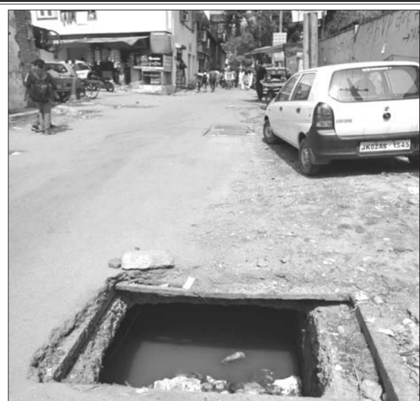
Gaping manholes dot Commerce College lane.
