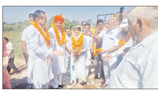
DDC Chairman Jammu, Bharat Bhushan kick starting blacktopping of Dharam Khu village road on Monday.
