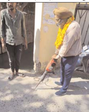
JMC Councillor, Inder Singh Soodan starting construction work of a bridge in Nanak Nagar.
