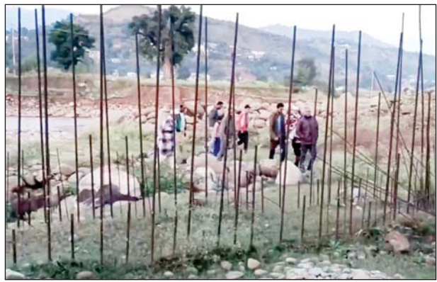
Construction work abandoned on a bridge since last 15 years in Mendhar area of Poonch district. -Excelsior/Rahi Kapoor
