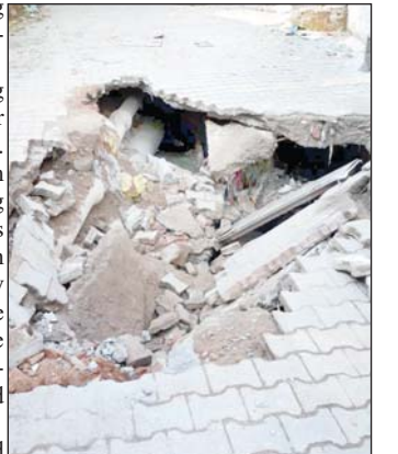
A lane caves in near Dakki Pir Kho in Jammu.
