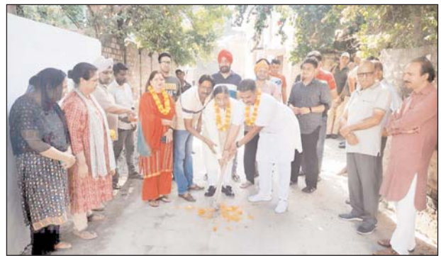
Former Minister, Sat Sharma and chairman JMC Hardeep Singh Mankotia kick starting construction of lanes and drains in Subash Nagar, Jammu on Thursday.
