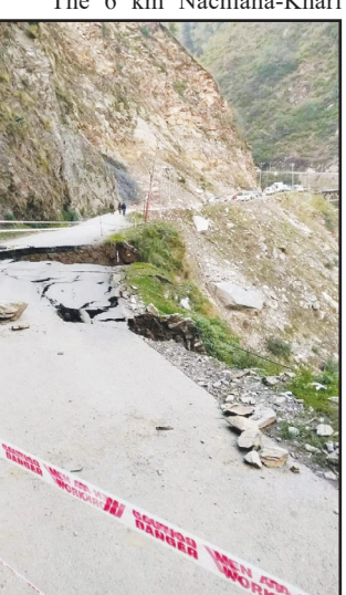
Damaged portion of Nachlana Khari link road in Ramban.
