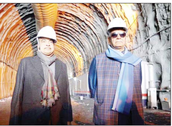
Union Minister of Road Transport and Highways Nitin Gadkari and Lt Governor Manoj Sinha at Zojila Tunnel to inspect the ongoing work on Monday. (UNI)
