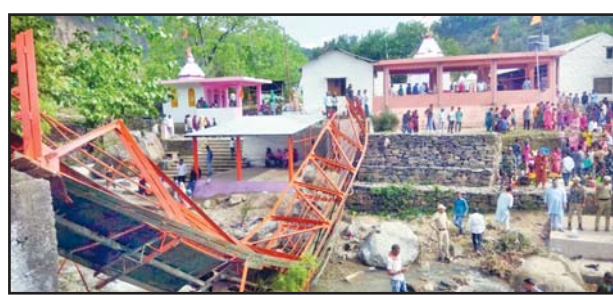
Collapsed footbridge at Beni Sangam in Chenani.
