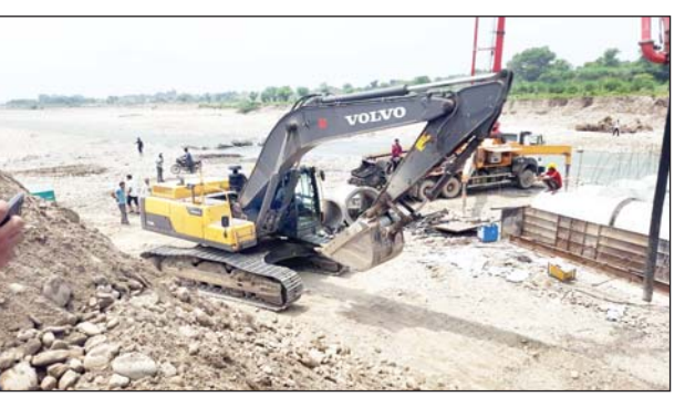
A machine on the job at Tarnah river to construct causeway for restoration of traffic on NH.
