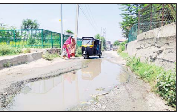
View of a dilapidated road near Islamia College leading to Makhdoom Sahib's Shrine in Srinagar on Wednesday.
