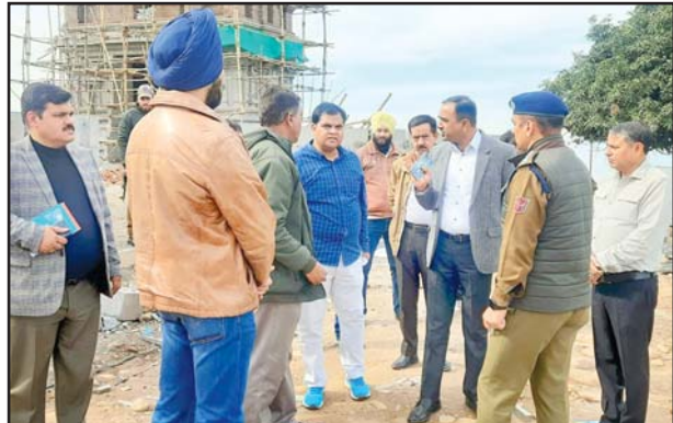
Div Com Ramesh Kumar during a visit to Tirupati Balaji Temple construction site on Wednesday.
