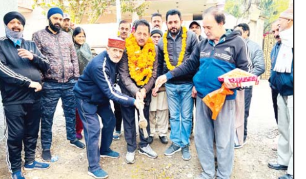
Dy. Mayor, Baldev Singh Billawaria starting work of laying tiles and construction of drains in Ward 56.
