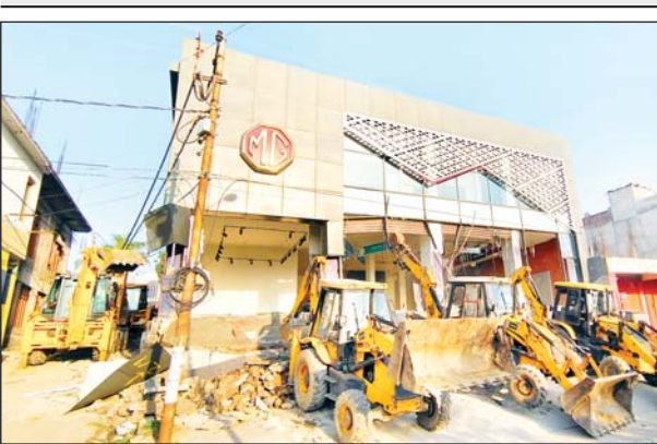
JCBs demolishing MG Hector showroom at Narwal, Jammu. Another pic on page 13.
