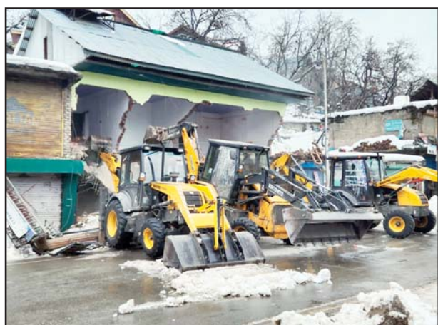
Commercial structure of former Social Welfare Minister Gh Hassan Khan on State land demolished by Revenue authorities in Shopian town. — Younis Khaliq
