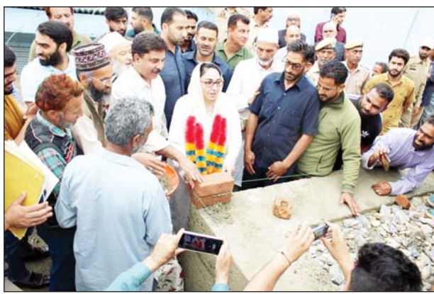
Waqf Chairperson, Dr Darakhshan Andrabi laying foundation stone for utility complex at Charar-e-Sharief.
