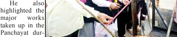
Sarpanch, Panchayat Kotli Shah Doula, Badrinath Sharma starting blacktopping work on Tanda road.
