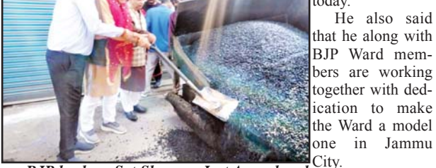
BJP leaders, Sat Sharma, Jeet Angral and others starting road blacktopping work in Ward 12.
