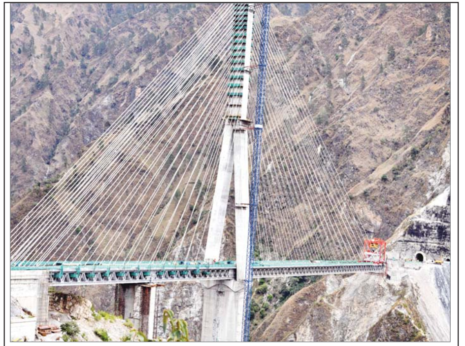
Construction work underway at Anji Khad bridge, India's first cable-stayed railway bridge, during a media preview in Reasi district on Sunday. (UNI)
