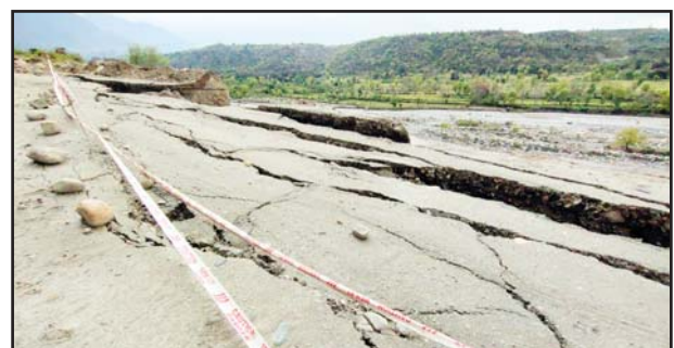
Sula Park-Baradhari Road in Reasi district damaged due to continuous rainfall on Saturday. More pics on page 10. — Excelsior/Romesh Mengi
