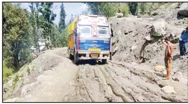
Dilapidated condition of a road in Doda.
